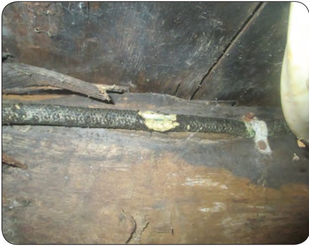
Figure 5. Rodent damage on electrical cable. Source: Heartland Farm Mutual, Waterloo, Ontario.
