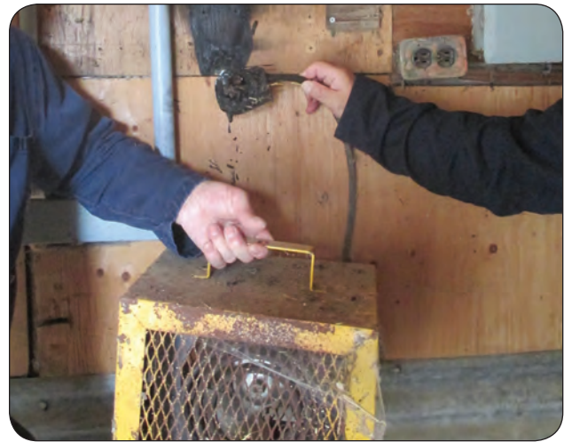
Figure 11. Fire started at box heater with receptacle and plug.
