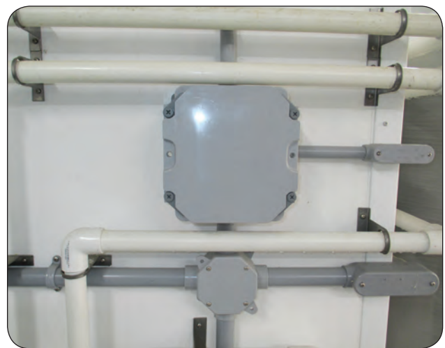
Figure 10. NEMA 4X rated enclosure. Source: Heartland Farm Mutual, Waterloo, Ontario.
