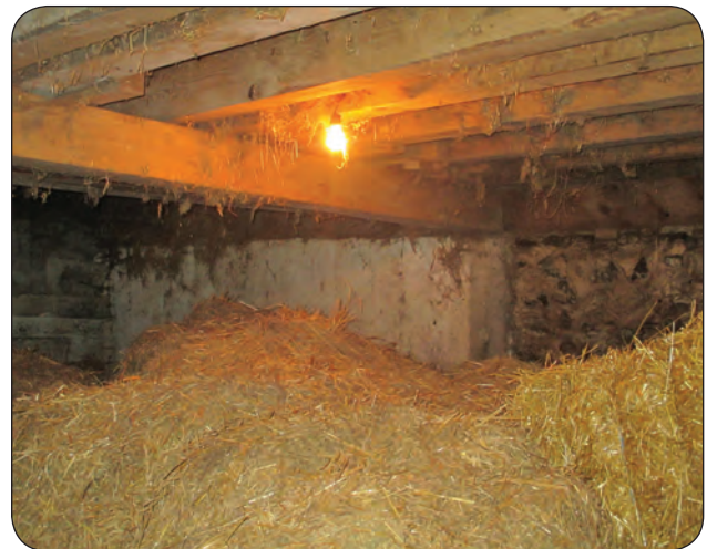
Figure 13. Flammable material near light fixture. Source: Heartland Farm Mutual, Waterloo, Ontario.
