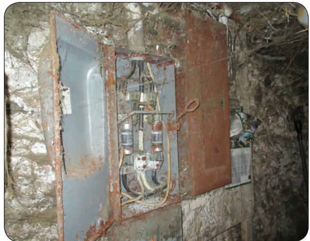
Figure 4. Corroded disconnect panel. Source: Heartland Farm Mutual, Waterloo, Ontario.
